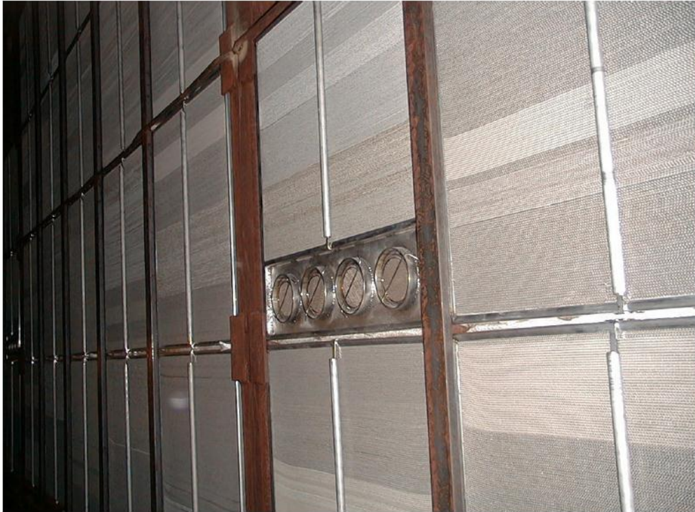
Figure 5. Monolithic Oxidation Metal Foil Catalyst Assembly (Source: Siemens HRSG O&M Plant Installation)
